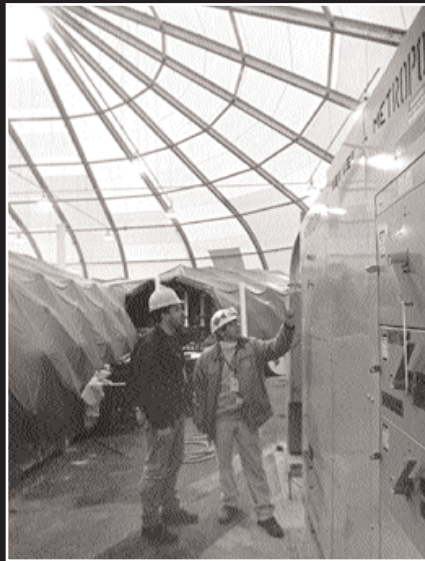
Electricians from Michael Mazzeo Electric Corp. examine a transformer at the EPA decontamination station.
