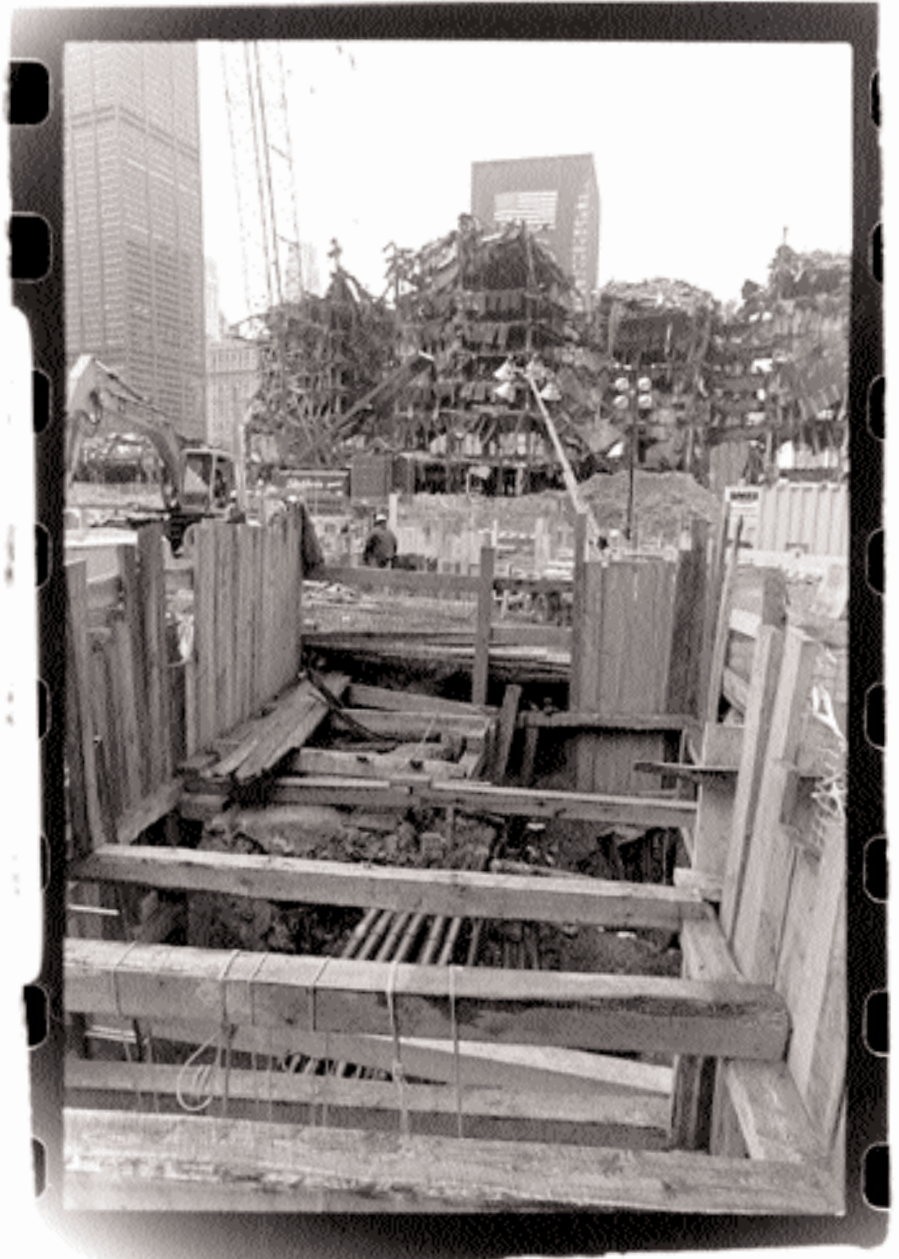
Temporary wiring running to 140 West Street.
